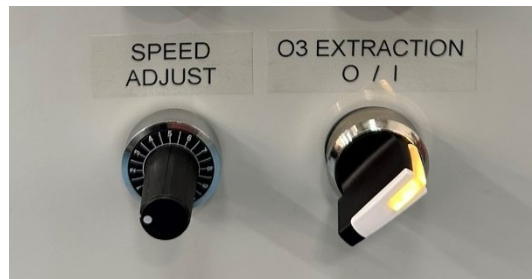
Ozone Extraction Alarm (Yellow)
